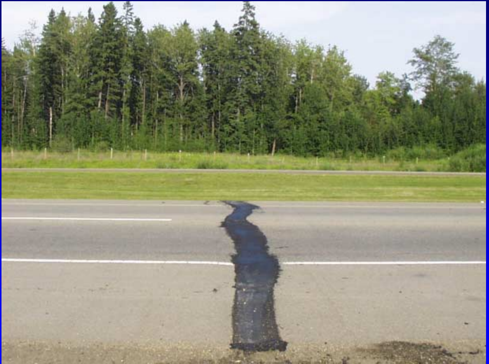
Transverse Crack in Styrofoam Insulated Pavement, Edmonton, Alberta
