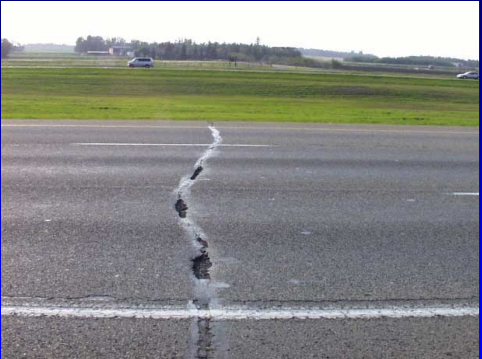
Deterioration at Transverse Crack
