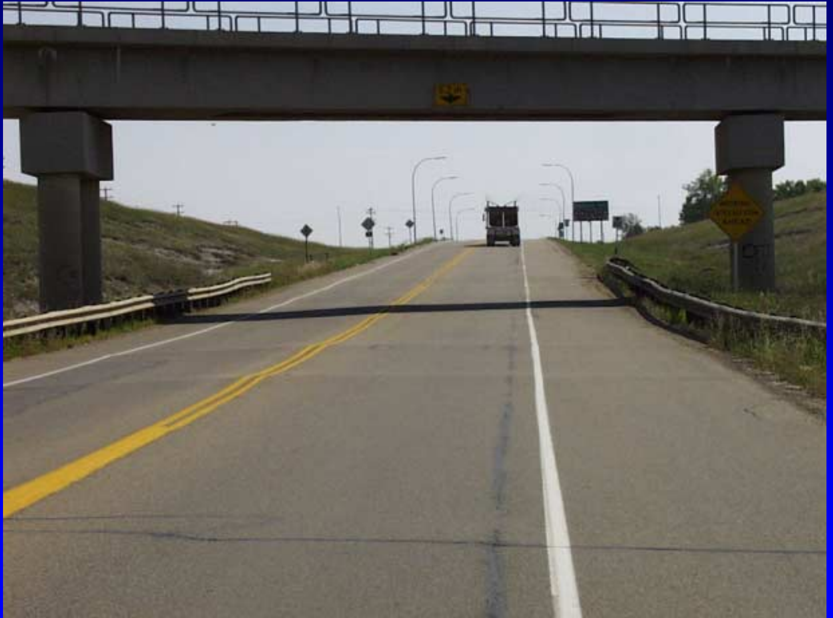
Heaving at Transverse Cracks
