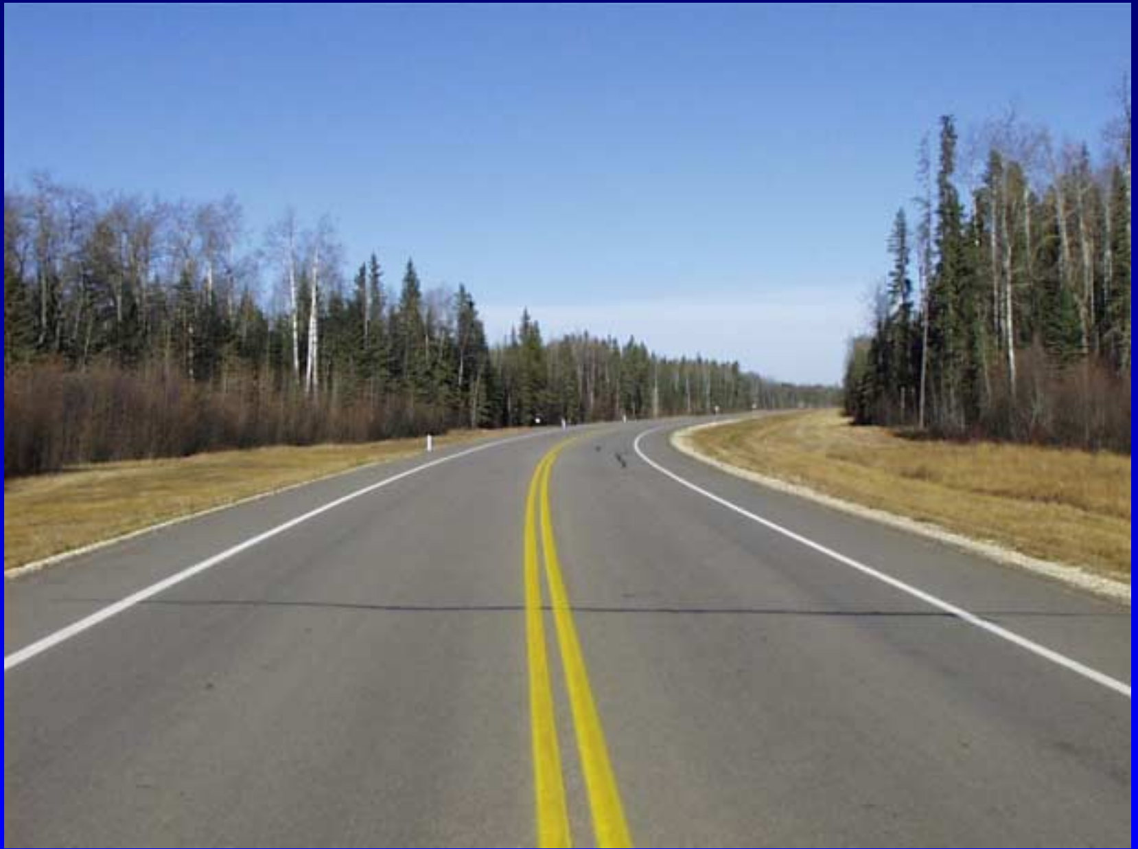
SH 813 (NE of Edmonton, Alberta) - Infrequent Transverse Cracking After 3 Years
