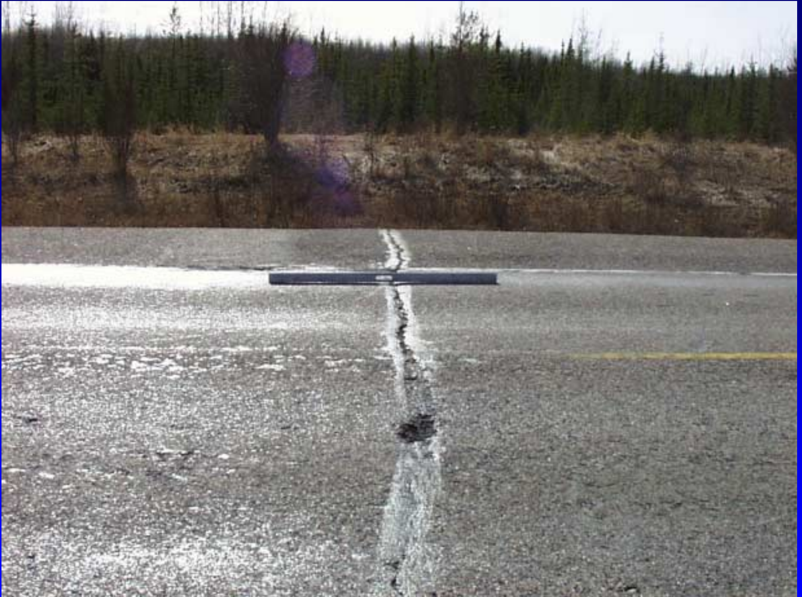
Dipping at Transverse Crack
