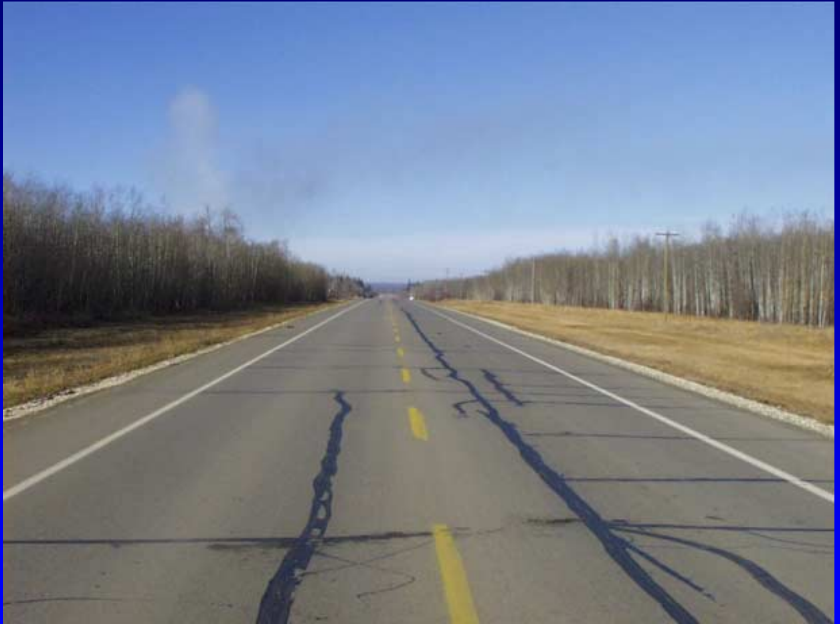
SH 813 (NE of Edmonton, Alberta) - Significant Transverse Cracking After 3 Years
