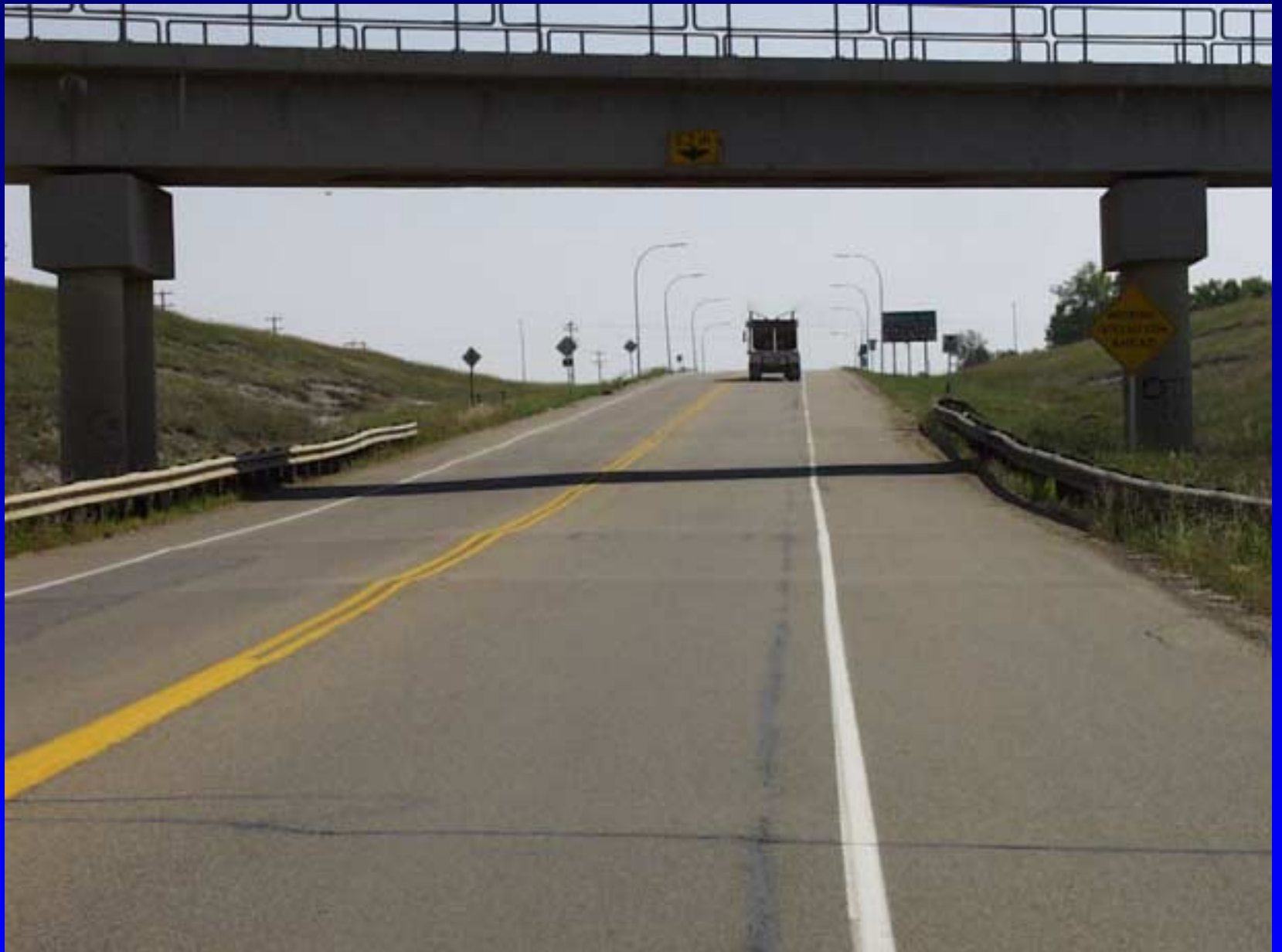
Heaving at Transverse Cracks
